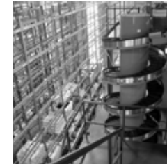
Warehouse Automation Systems
